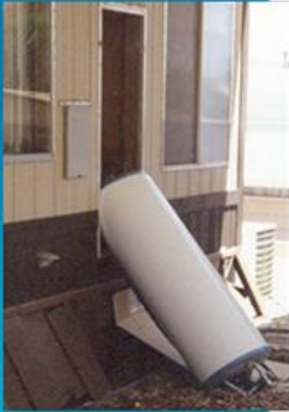
During an earthquake, an unbraced water heater can topple, which can start a fire or lead to major water damage.
