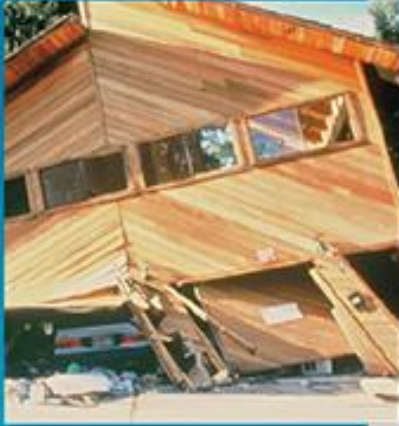
The walls around the garage door of this home were not strong enough to withstand the shaking of the 1989 Loma Prieta Earthquake.
