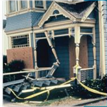
This older home collapsed after earthquake shaking damaged its crawl space (cripple) walls.
